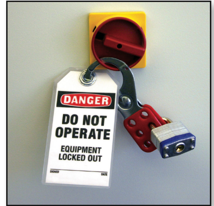
Locked out and tagged out (LOTO)
