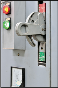
Main disconnect switch
