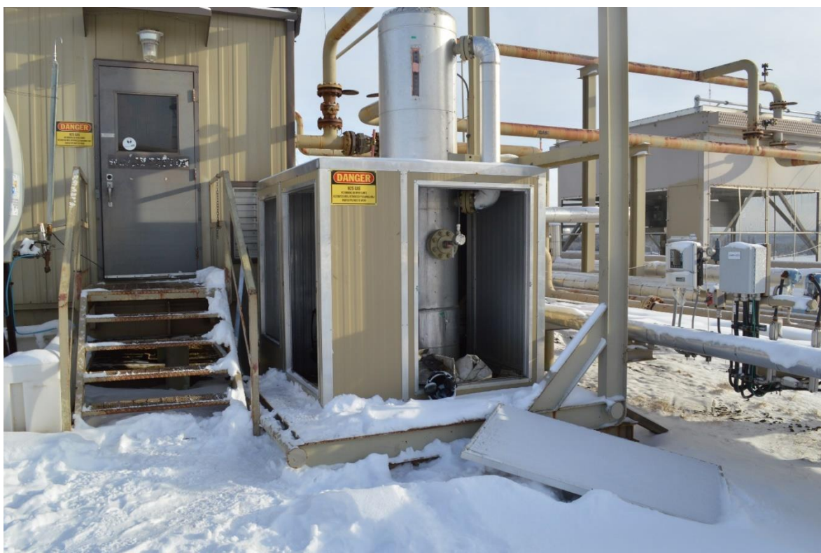
Figure 1. Utilidor cyclone separator where Operator 1 was found.
