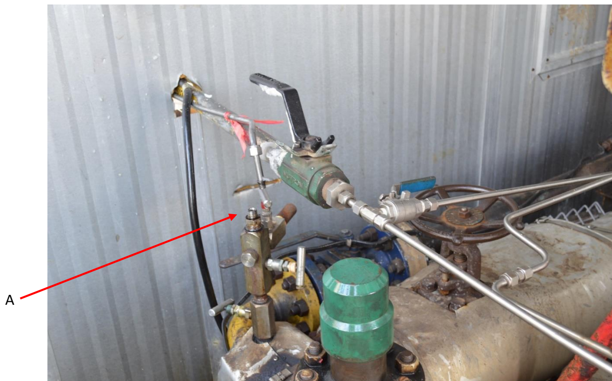
Figure 5. Valve Operator 1 was working to unblock.
